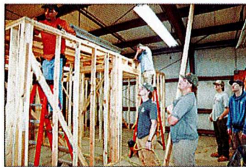
Students in East Mississippi Community College's Construction Engineering Technology class frame walls that will be used for an electrical training program at The Mission in West Point. The program aims to give men at the residential treatment facility the skills they need to enter the career field or continue their education.
