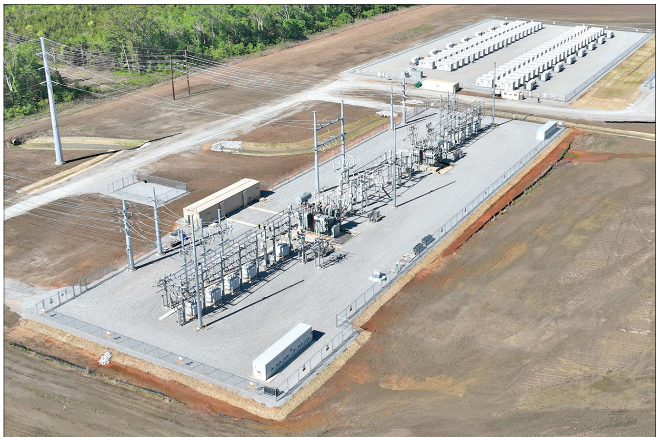
The Golden Triangle II battery bank and substation is pictured. The site, which began operating in May 2024, is one of four solar projects Origis Energy has brought to the Golden Triangle region through the Tennessee Valley Authority’s Green Invest program. The increase of solar projects in the region reflects a bigger push by the TVA to add up to 10,000 megawatts of solar to its electrical grid by 2035.
