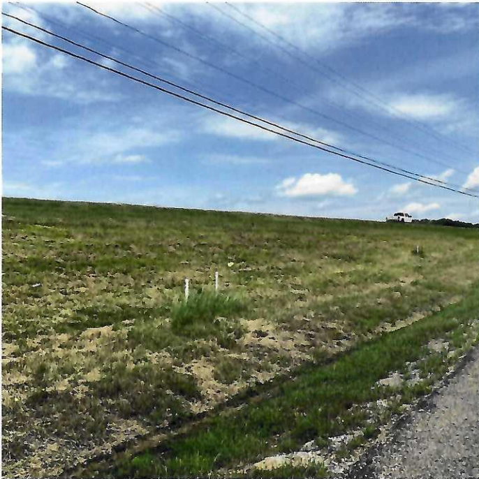
PHOTO 7 —Downstream slope view from left side of dam (Utility lines visible and 3 of 5 piezometers)
