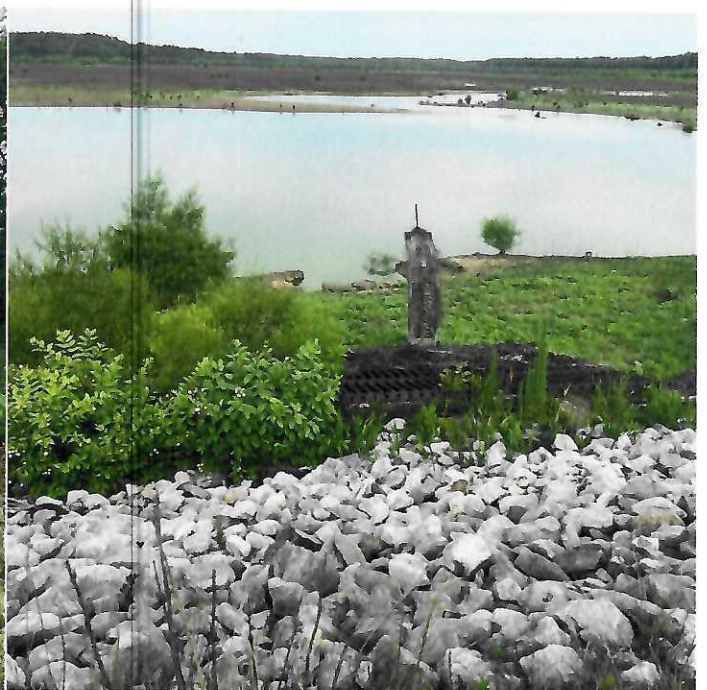
PHOTO 4—Primary spillway (note missing riser)
