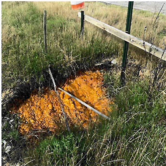
PHOTO 11 — Area above primary spillway where sinkhole opened caused by joint separation
