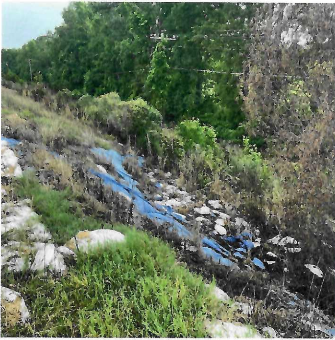
PHOTO 13— Slide area along downstream right embankment
