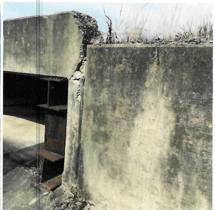
PHOTO 16— Structural damage at downstream left corner of auxiliary spillway
