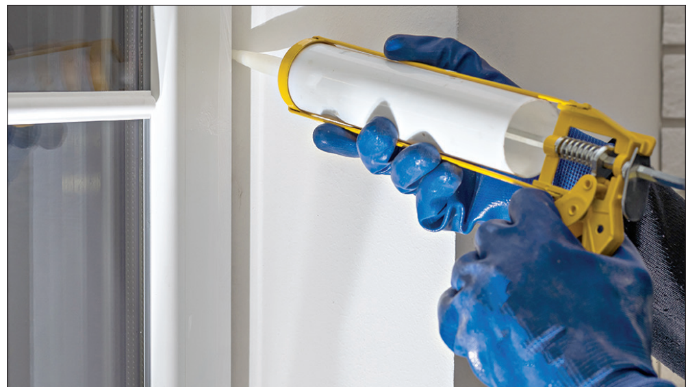
Stock photo Caulking around your windows and doors conceals gaps to make it easier for the air in your home to stay at the right temperature for the season which can lead to energy savings.
