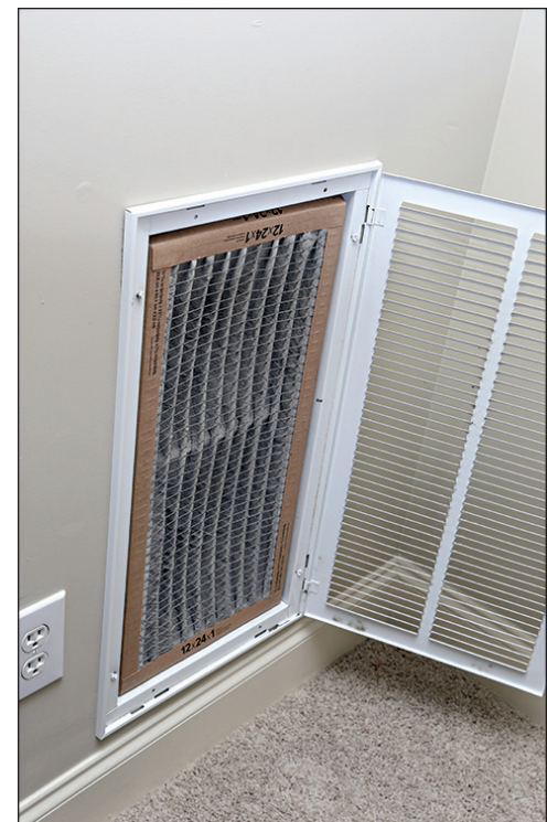
Stock photo Replacing a dirty, clogged filter with a clean one can lower your air conditioner's energy consumption by 5% to 15%.
