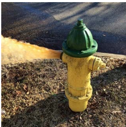
Picture of Ward 5 Hydrant Flush
